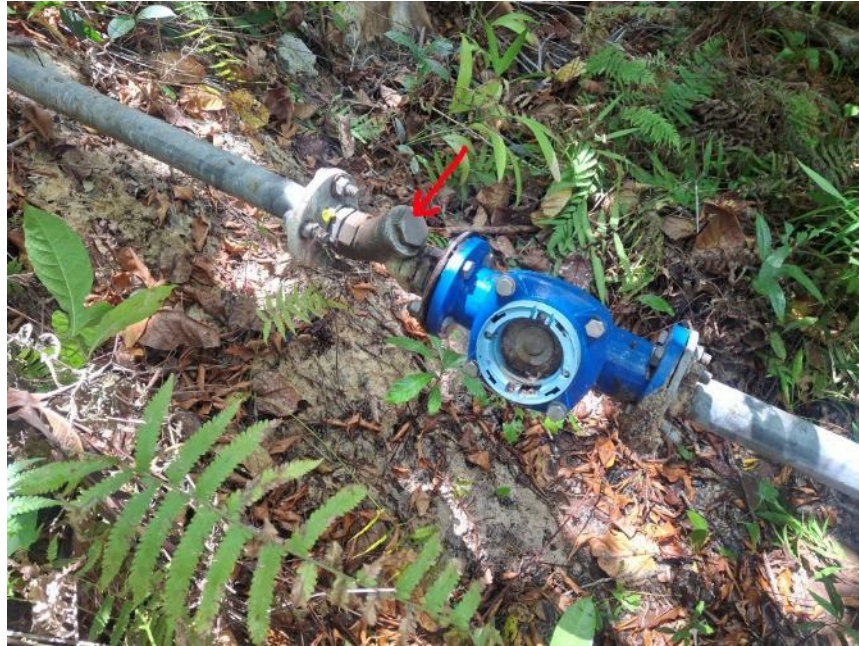
The in line filter cleaned out of much rubbish of leaves & twigs. (The filter is contained under the large bronze nut indicated by the arrow)
