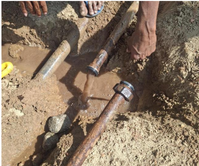
Supply pipe from big tank located and opened at barrel union (joiner). Note the degree of dirt coming from the pipe.
