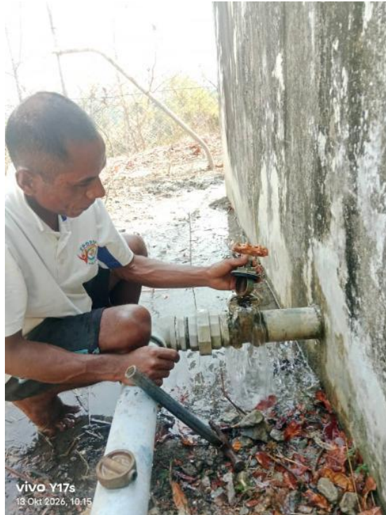
Water pouring out of gate valve with broken tap-head.
