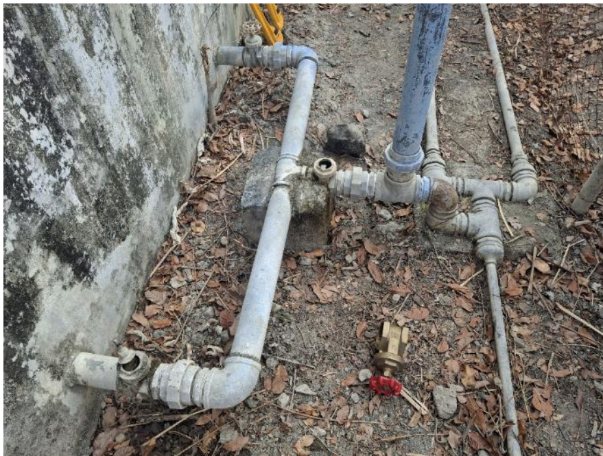
This is the exit pipe network from big tank. Note two of the gate valve tap-heads are broken.
