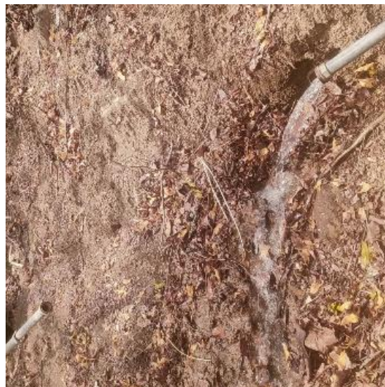
Near-vertical section of hill, pipes not correctly aligned; joint broken, pipes slid apart.
