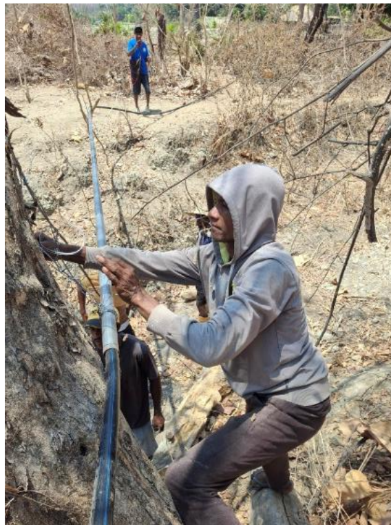
32mm poly pipe encased in a gal pipe for strength, and suspended well above a creek on the western bank.
