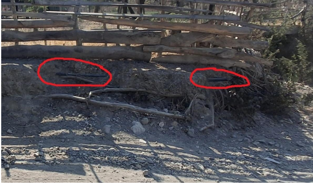
Old pipe on western bank – exposed and torn apart by flooded river. This was the only section found in the 600m from the aerial ropeway! (Red ovals show ends of the pipe)
