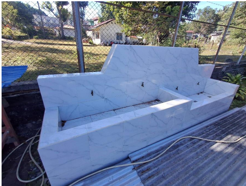
Hand washing station at front of hospital, which was not connected to a water supply. It is now connected. (Built originally by UNICEF)
