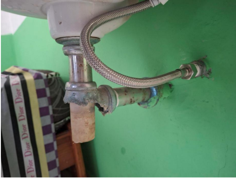
Flexible hose replaced, but drain needs replacing. (Staff are using a temporary bucket.)
