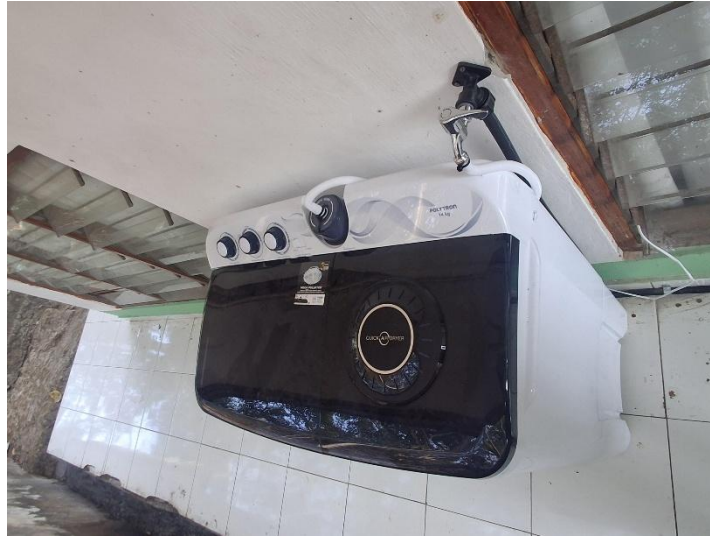
New washing machined donated by John Flood – for use by maternity ward for washing bed sheets etc
