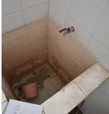
Water tank in maternity ward from which water is normally scooped to flush toilet. Tap broken.
