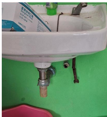
Handbasin in nurses' room. Tap missing handle; flexible line not connected & broken; drain pipe broken off
