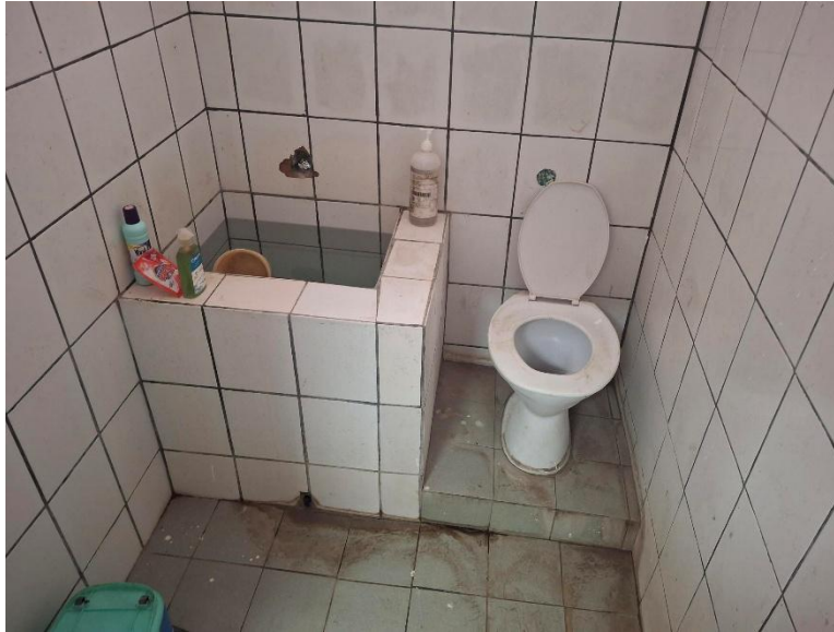
No tap over water tank, but stick inserted to stop flow. Stick was removed to fill tank. Water is scooped from tank with pink bucket to flush toilet.
