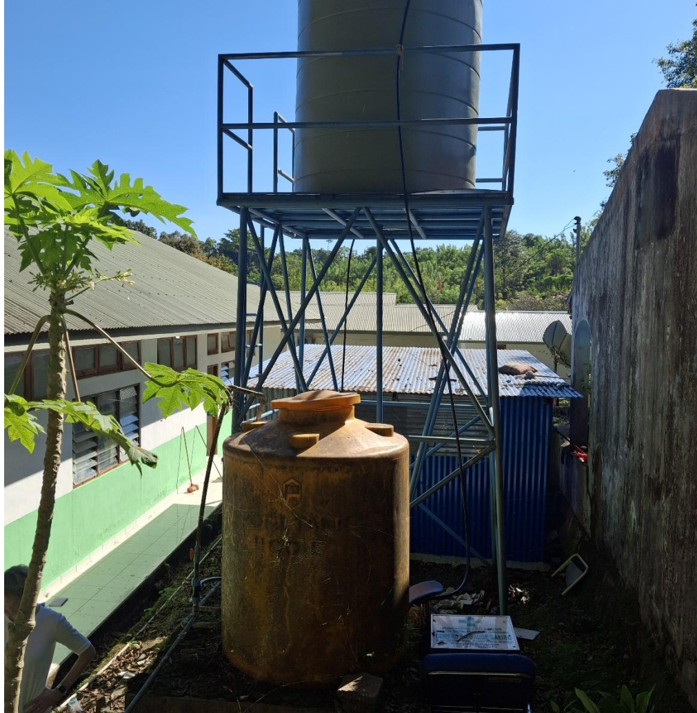
Existing tank stand, with recently installed (not by us) 5,200 litre tank on top. Dirty yellow tank in front will be replaced.
