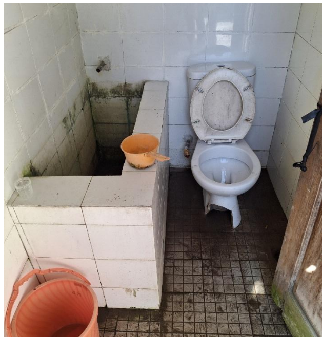
A toilet in the outside area used by the public. No tap over the tank, and no tap and pipe supplying water to the cistern. Toilet bowl broken. Floor filthy and very smelly.
