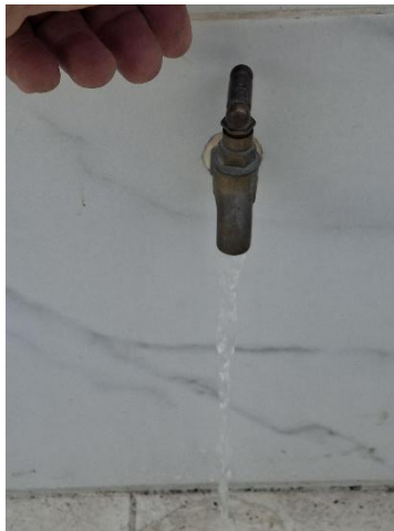
Water flowing at hand washing station
