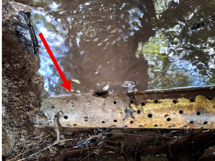
Large hole in entry strainer pipe (red arrow) and inlet holes blocked below water line
