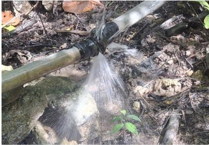
Ineffective tyre inner-tube joint
