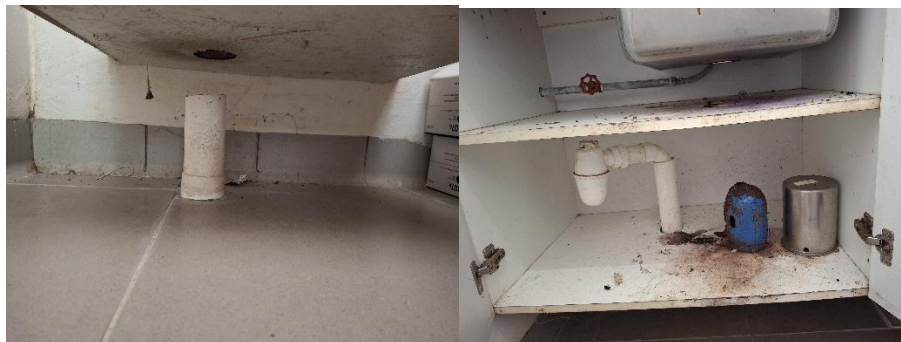
Basin drains not connected
