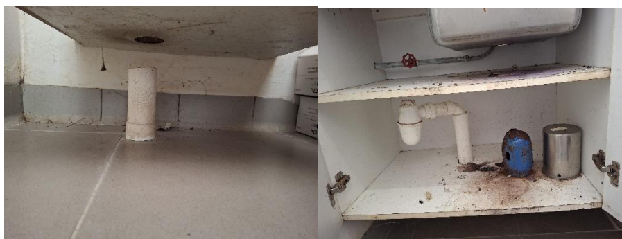
Basin drains not connected
