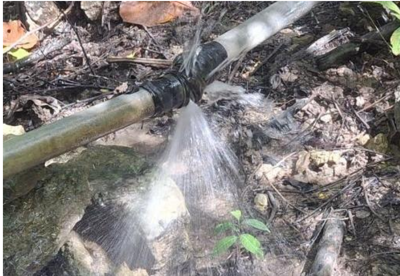
Ineffective tyre inner-tube joint
