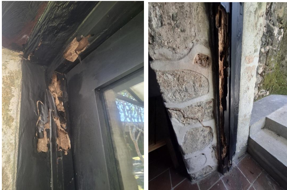
Severe white ant damage in door frames at the Museum
